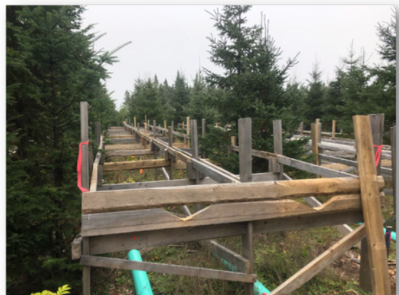
Image 2. Eavestroughs repaired and reinforced with additional wood, without tarps. Photo: Chloe Larstone Hunt, 2023
